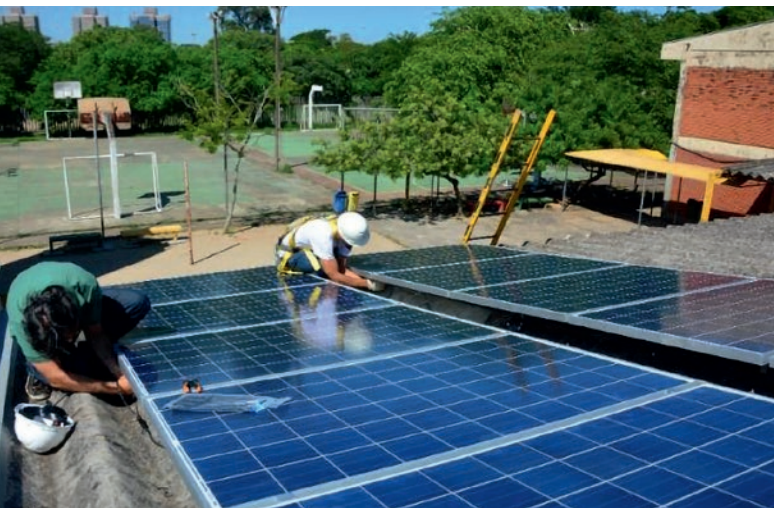
Porto Alegre's pilot PV installation in one of the municipal schools.
