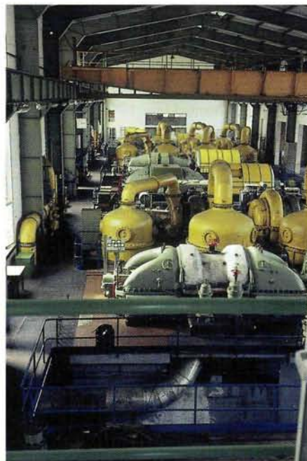
Geothermal power station in the Latera area (Latium) in Italy
