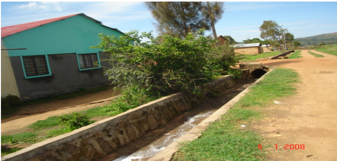
Fig 4.5: Stone Linen Drainage which is border between the airport and Bangwe Settlement.
