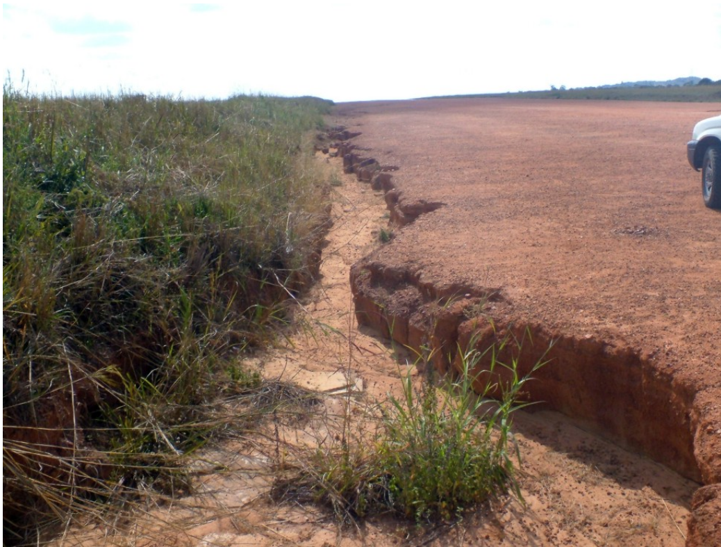
Fig 6.1: Soil Erosion along the Runway
