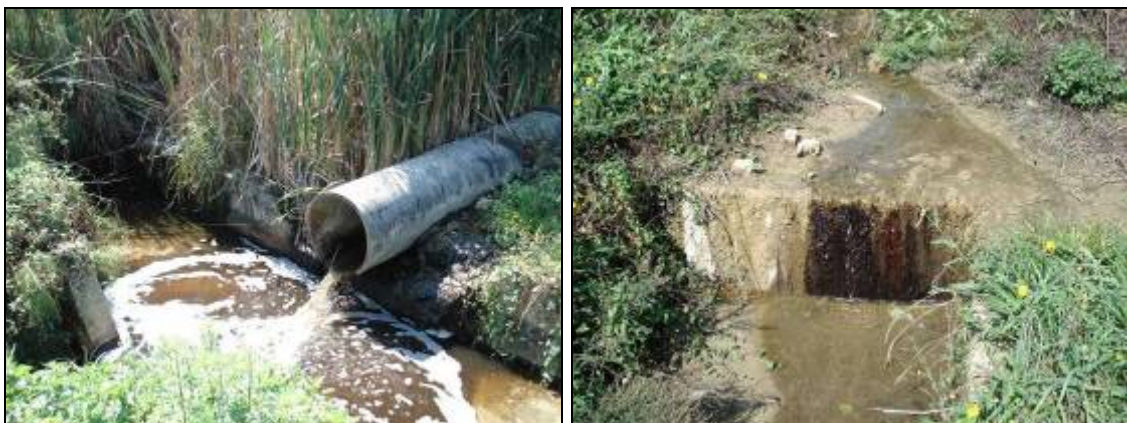
Picture no. 24 Main sewer under the dam of the Ramići existing landfill
