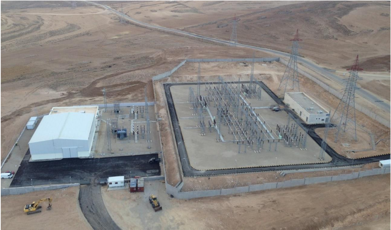
JWPC and NEPCO substation
