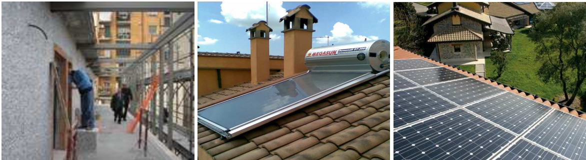
Figure 23 – From left: installation of thermal insulation on an existing building, solar panel on the roof of an existing building, photovoltaic panels on the roof of an existing building.
