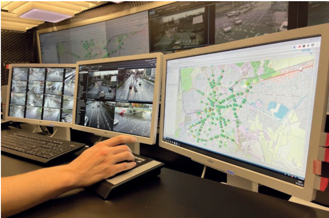
Timișoara traffic management command centre. Source .
