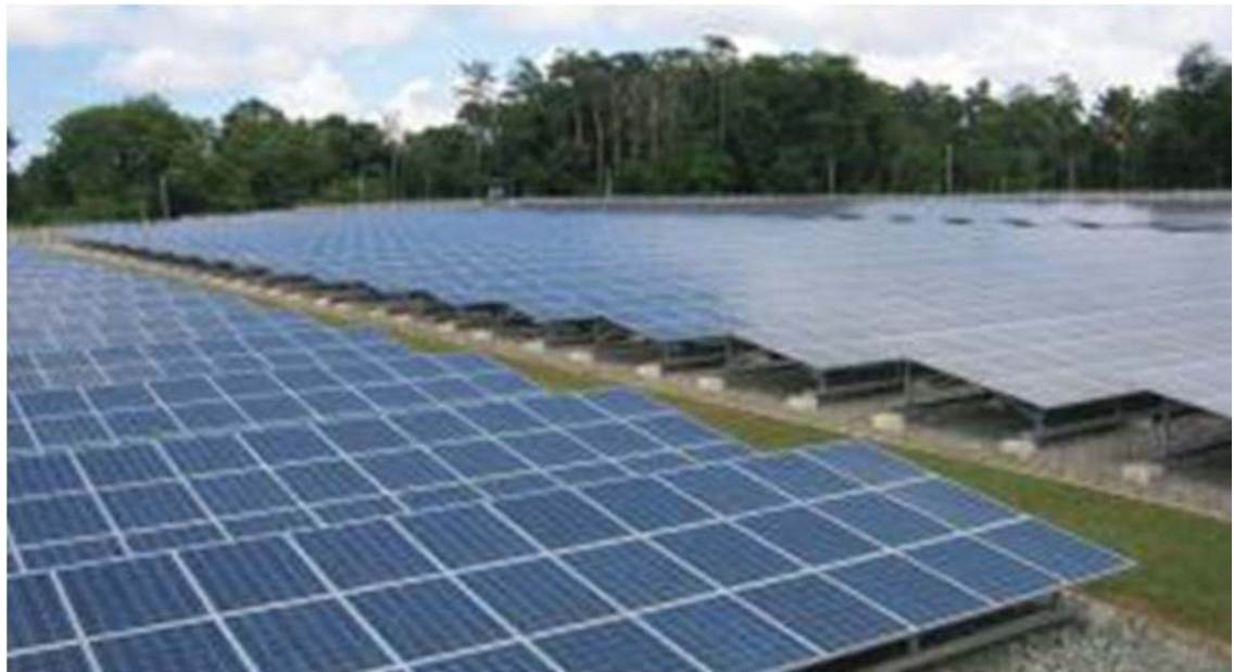
Typical Installation of Solar Modules
