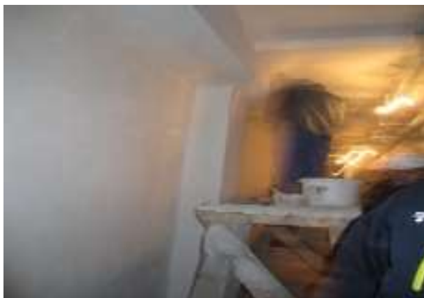
Figure 13: Work at height without safety belts by construction contractor personnel at Peremoha station
