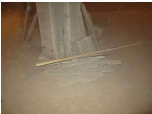
Figure 15: Use of asbestos materials at Peremoha station
