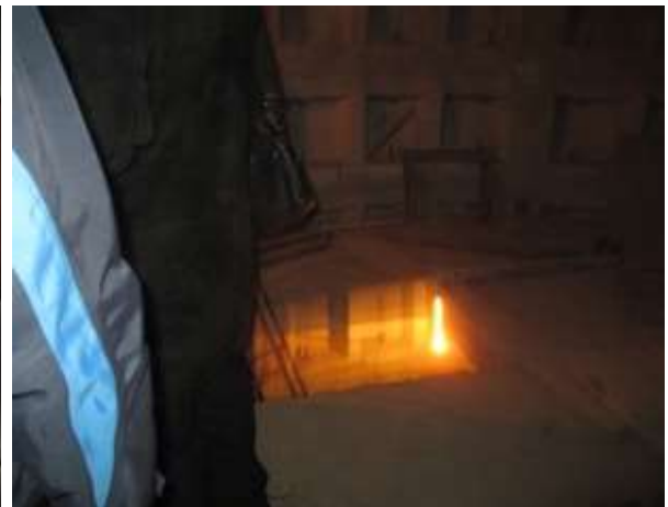
Figure 12: Openings were not fenced. Poor lighting of workplaces at Peremoha station.
