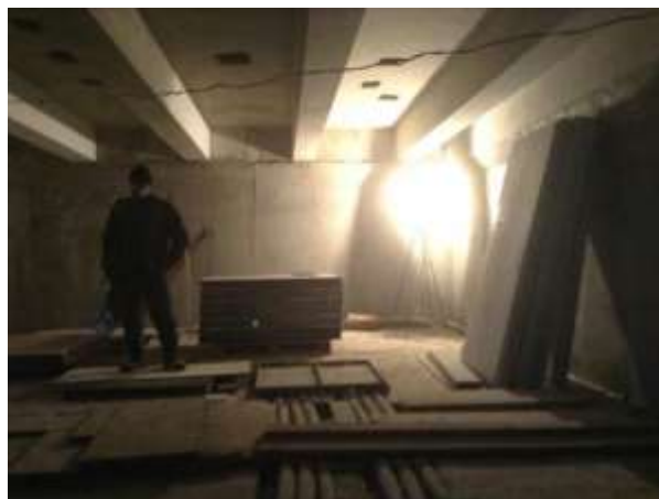
Figure 16: Use of asbestos materials and lack of appropriate PPE by construction contractor personnel at Peremoha station
