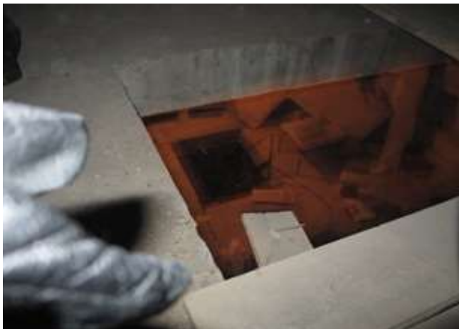
Figure 11: Openings were not covered at Peremoha station
