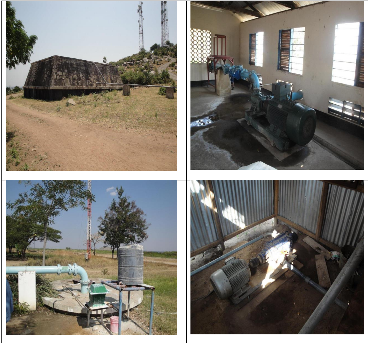
Figure 2-2. Some of the existing water supply infrastructures
