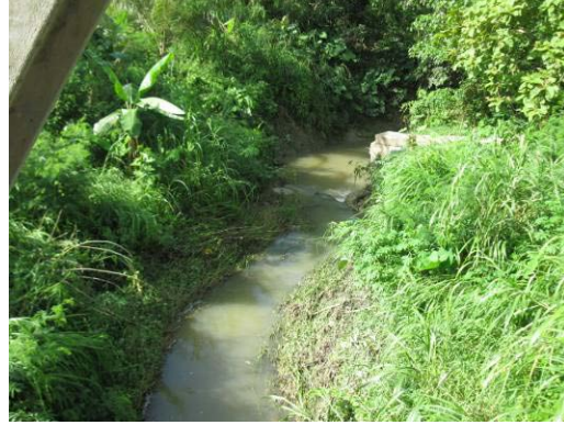
View downstream showing remains of the old abutment
