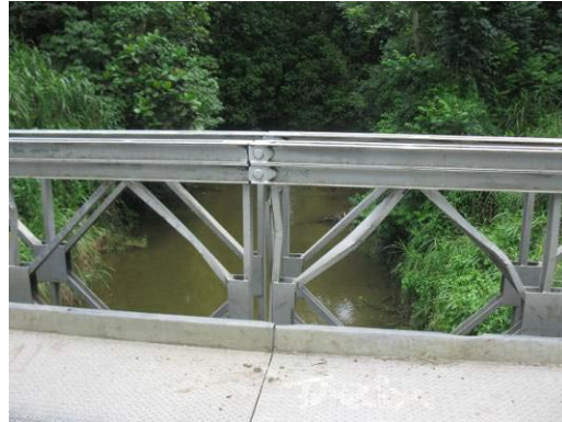
Deformed diagonal member of panel
