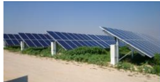
Figure 4: Aerial view of solar PV panels installed in an SEF
