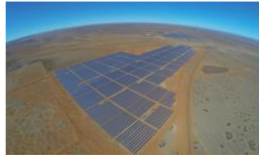
Figure 3: Fixed solar PV panels installed in a SEF
