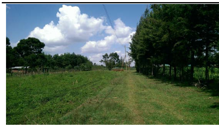
Figure 7.3 Overhead Electricity Distribution Lines Observed in Mosop Village
