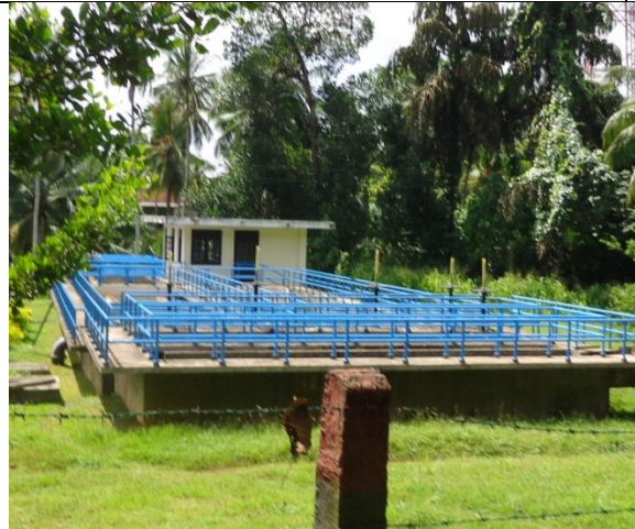
Figure 12 settlement [pond at the BOI Facility
