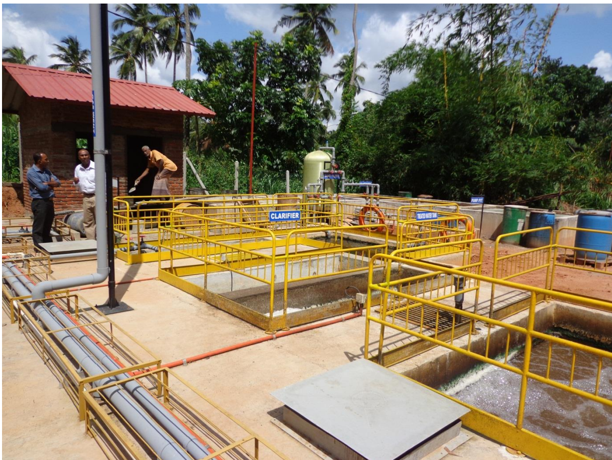
Figure 22 Existing Water Treatment Plant at SMG Coconut Processing Plant
