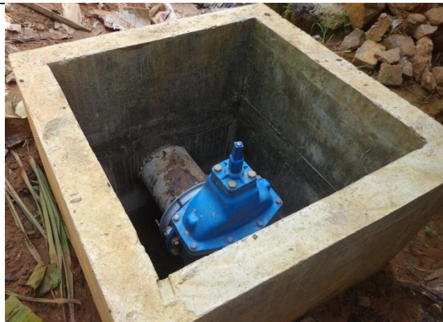
Figure 15 Main distribution valve
