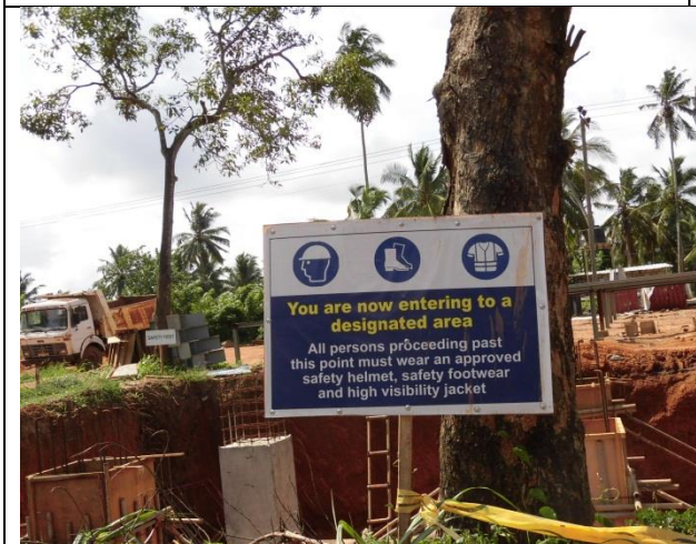
Figure 19 Some of the construction sites not protected properly
