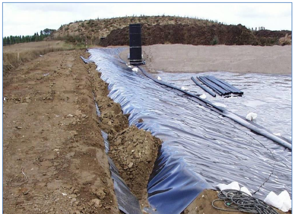
Figure 2.5 Construction of waste disposal cell, with bottom clay layer, HDPE liner on bottom and slopes, and a leachate collection well at the lowest point of a landfill cell
