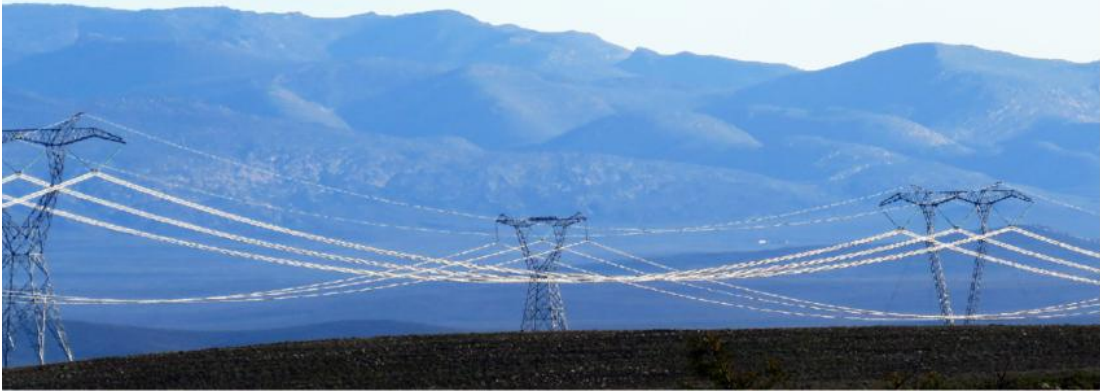
Figure 1. Example of 400 kV and 220 kV transmission lines constructed in parallel with staggered towers.
