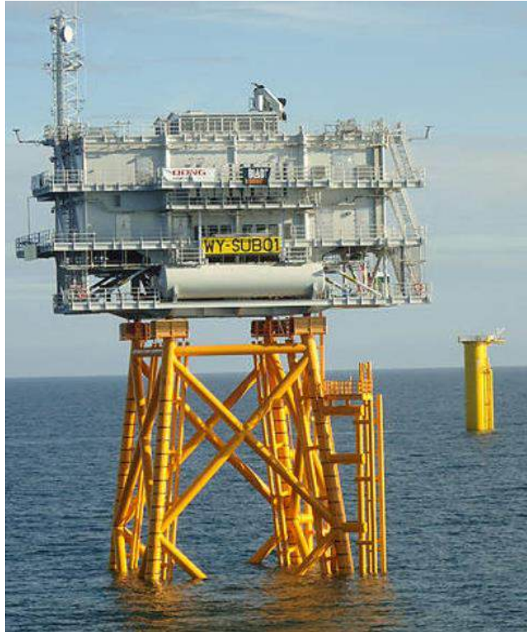
Figure 2.10. Offshore substation at Walney Phase 1 OWF [Source: https://www.isc.dk/en/walney-i-ii-vindmoellepark/ ]
