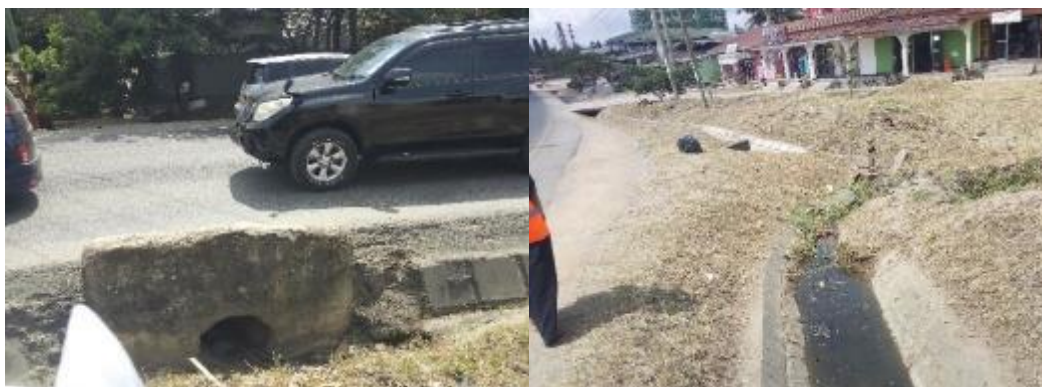
Figure 4-28: Storm water drainage system along Tabata- Segerea section
