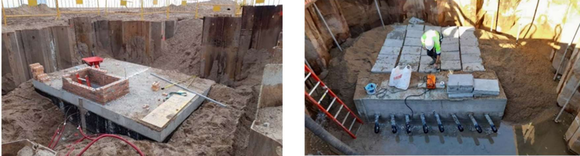
Figure 3. Example of BMH (left) and border pipe (right) infrastructures. Source: AFR-IX Telecom.
