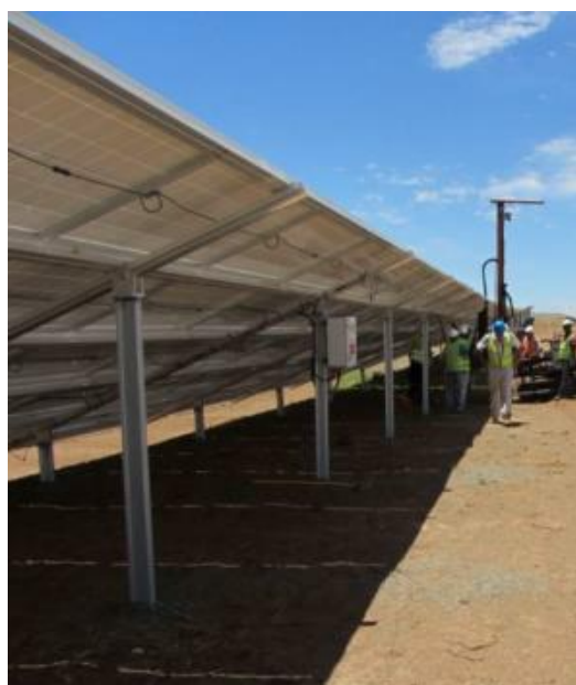
Figure 2-6. Example of fixed tilt solar panels on H-style steel piles
