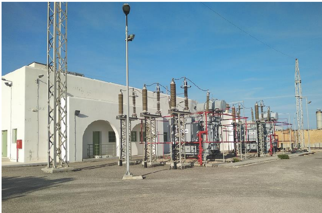
Figure 6-7. Typical view of substation GIS 150 kV/MT Paros
