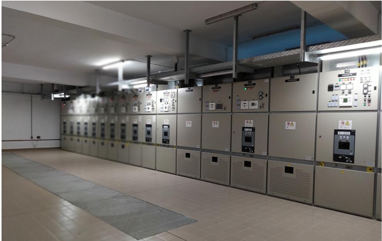
Figure 6-6. Typical view of 20 kV GIS average voltage tables at 150 kV/MT substation
