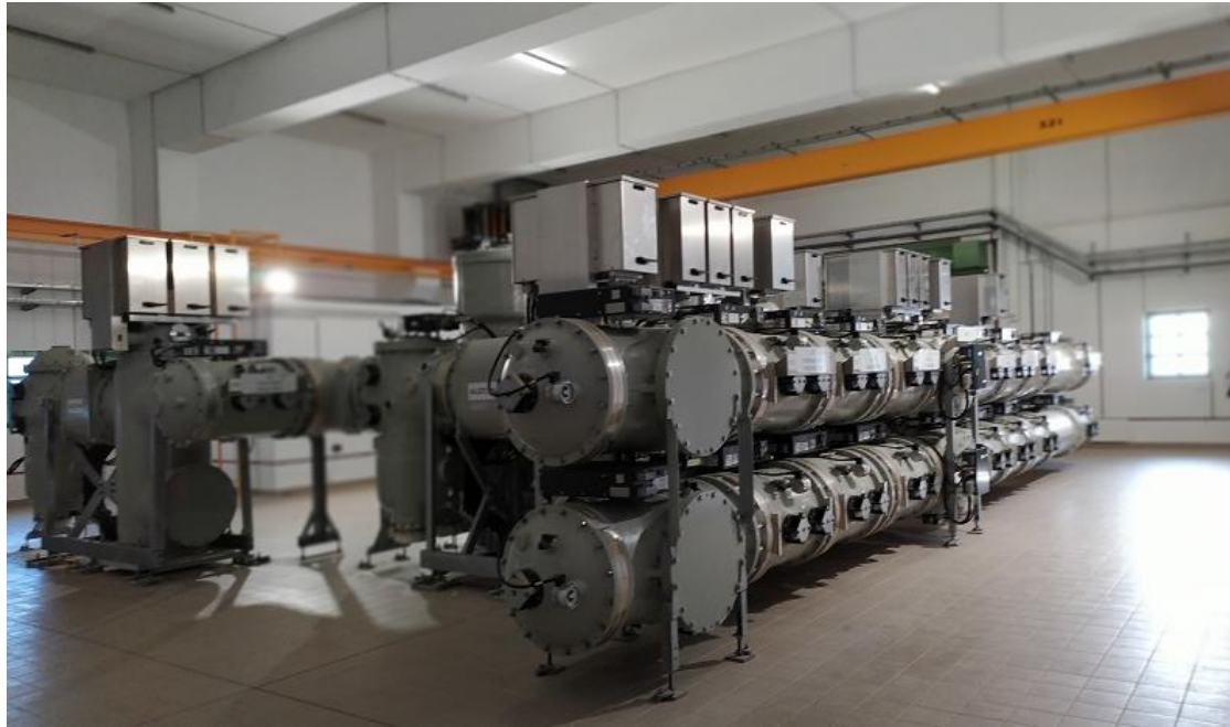
Figure 6-4. Typical view of 150 kV GIS balances and gates at 150 kV/MT substation
