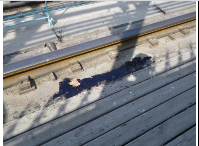
Picture 8 – The crane leaks.
