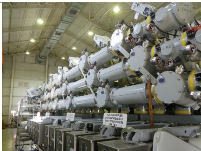
Picture 3 – New switch at the switchyard, financed by ADB.
