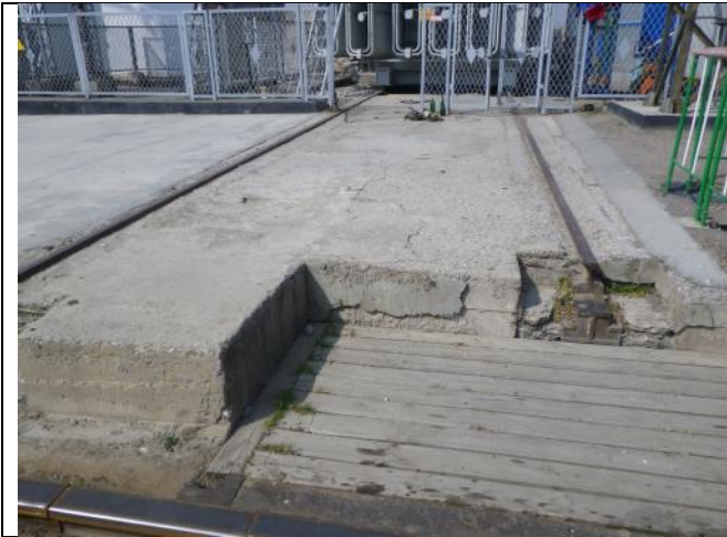
Picture 7 – Overall resurfacing is required on the dam crest.
