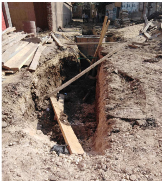
Figure 12: Collapse of trench in one IWSP 1 project
