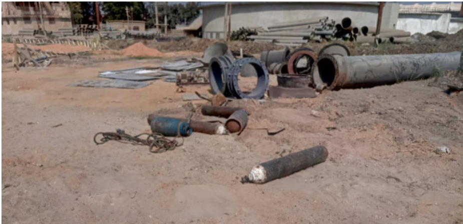
Figure 13: Acetylene cylinders shattered all over the project site
