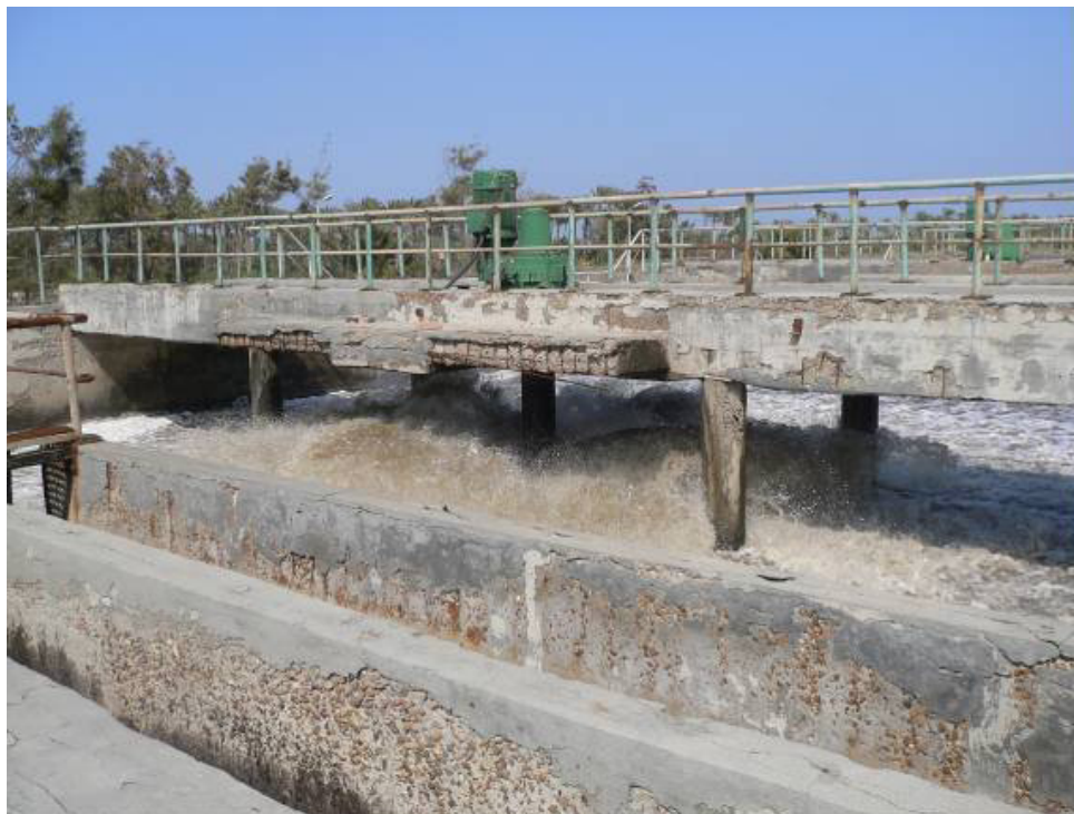
Figure 17: Aerators at Ras el Bar WWTP highly contribute to indirect CO 2 emissions and most probably to direct N 2 O emissions
