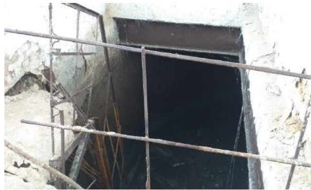
Sewage from nearby multi-storey buildings flows by gravity into the tank
