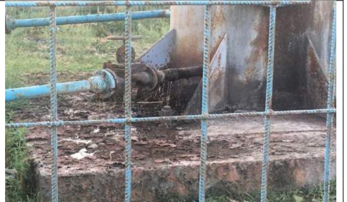
Water tower casings are worn out, tanks and supply pipes are leaking. Support structures are subject to corrosion
