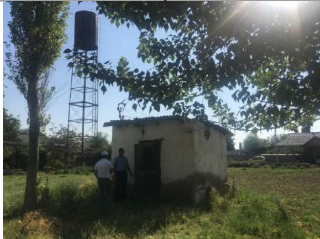
The water intake building needs to be repaired
