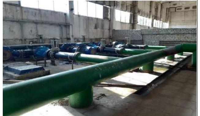
Wastewater pumping pumps to sewage treatment plant
