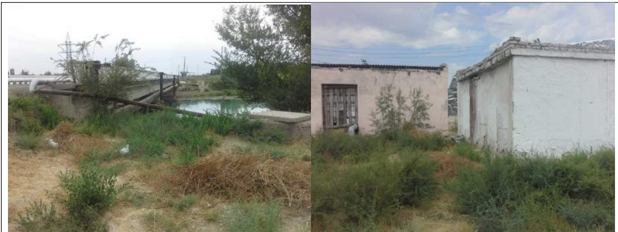
Wastewater of the village was pumped through the system "siphon" to the treatment plant in Yangier. In the right photo there is an inactive SPS, on the left there are remaining pipes, and on the far bank there is a sewage collection tank.
