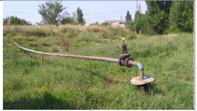
The pipes are rusted and leaking
