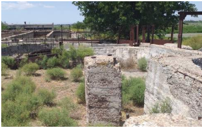
The sewage treatment plant was decommissioned in 2003 due to frequent flooding and the threat of contamination of nearby areas
