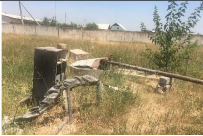
Deteriorated pipes leaving the water intake.
