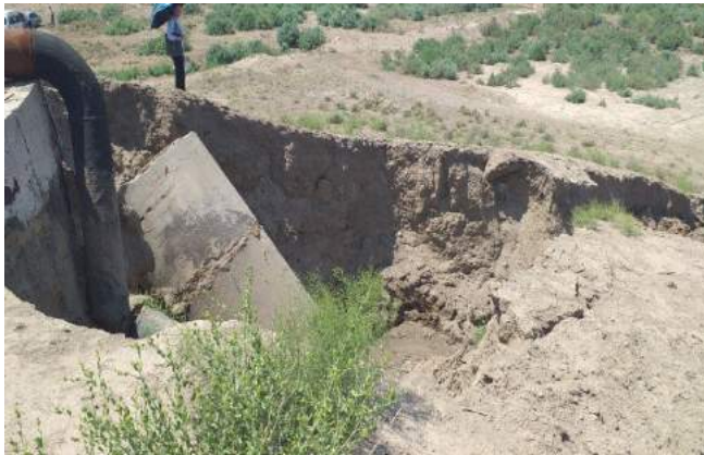
In 2018, a partial reconstruction of the STP was carried out. Unsecured soil supporting the supply pipeline was washed out and destroyed by runoff
