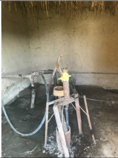
Worn-out equipment in the water intake building
