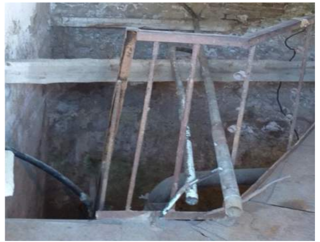
The building and equipment are in poor condition.
