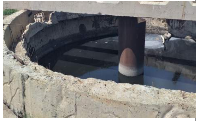
At present, waste water is discharged to nonoperating treatment facilities.
