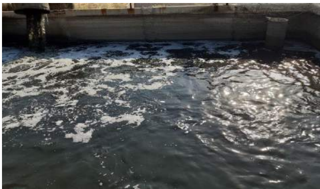
Due to the large deterioration of structures, water is not treated properly
