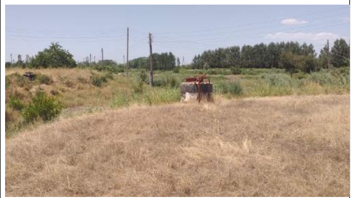
There are 4 underground water reservoirs on the territory of the intakes, two of which are not working. The total volume of tanks is 6000m 3
