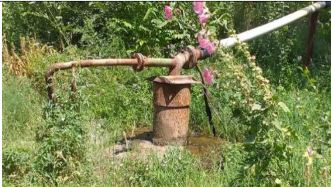
Water intake well on the territory of «T. Malik» mahalla. Provides water for several cottages and a hospital. The volume of underground water dries up, so that water is supplied in the evening for only 1 hour and 20 minutes.
