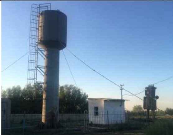
In most cases, the «Rozhnov's water towers» have been installed in rural areas.
