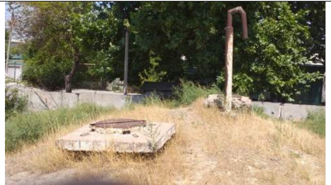
The underground tank capacity is 250 m 3 . The underground tank is cracked and needs to be repaired. Water treatment is not performed.
