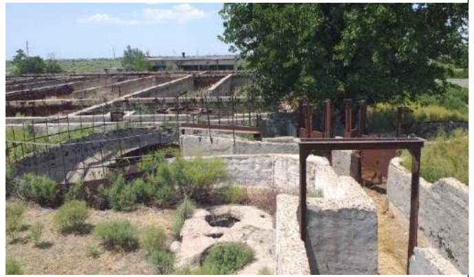
At present, there is a question about the disposal of massive reinforced concrete structures
