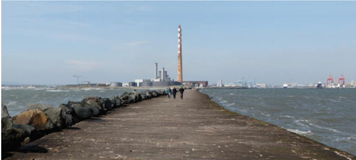
Figure 5 Construction Phase as seen from the South Bull Wall (tower cranes to the far left of the chimneys may be visible)
