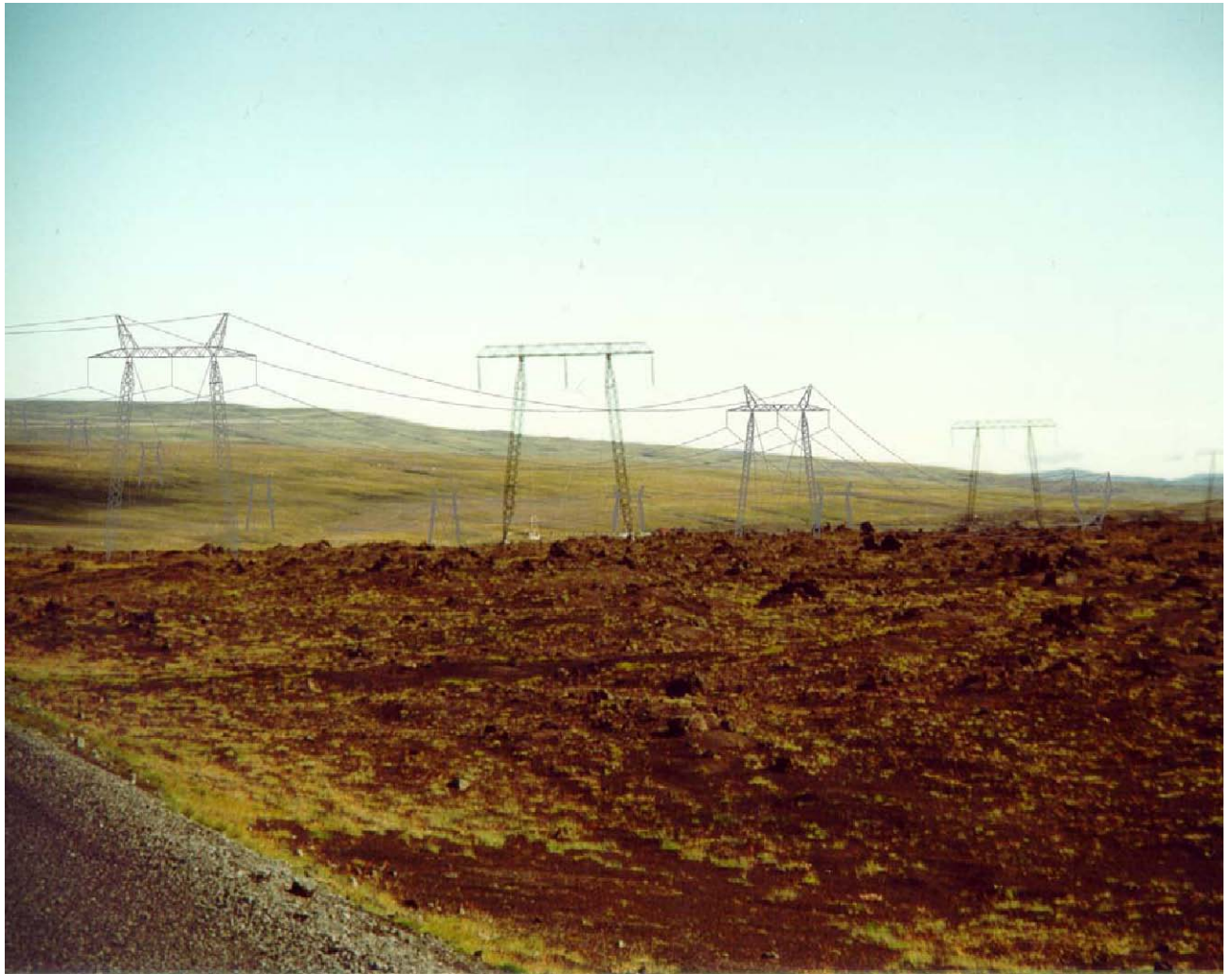
Fig. 5.5 Búðarháls line 1, looking north over Búðarháls from Highway 26, with Hrauneyjafoss line 1 in the foreground. Both the towers and the wires are indicated more clearly by having them a darker colour than they will actually be.
