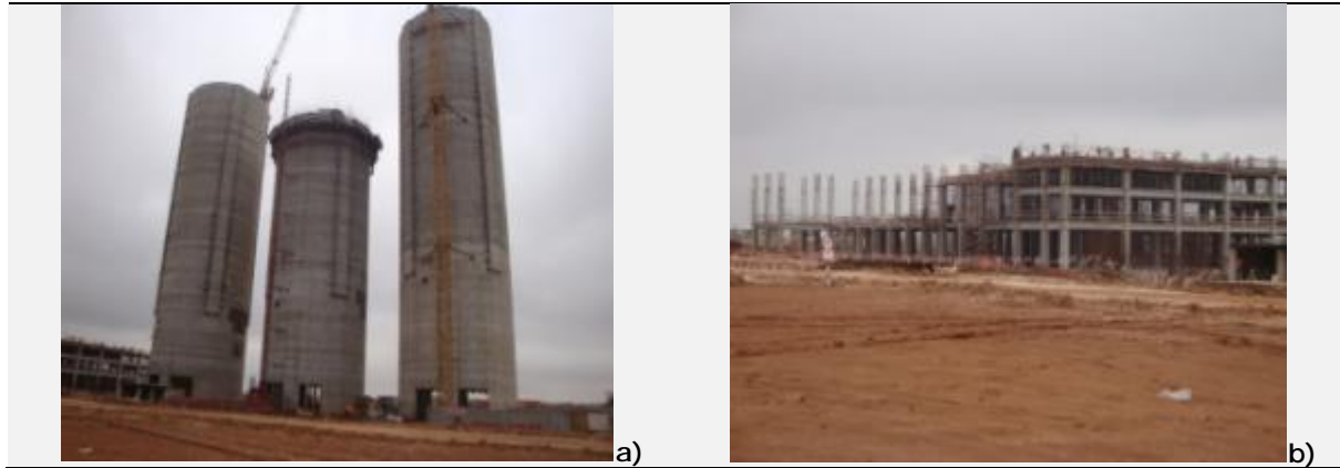
Figure 2-7 a) Cement Silos and b) Packing Plant under Construction at Plant Site
