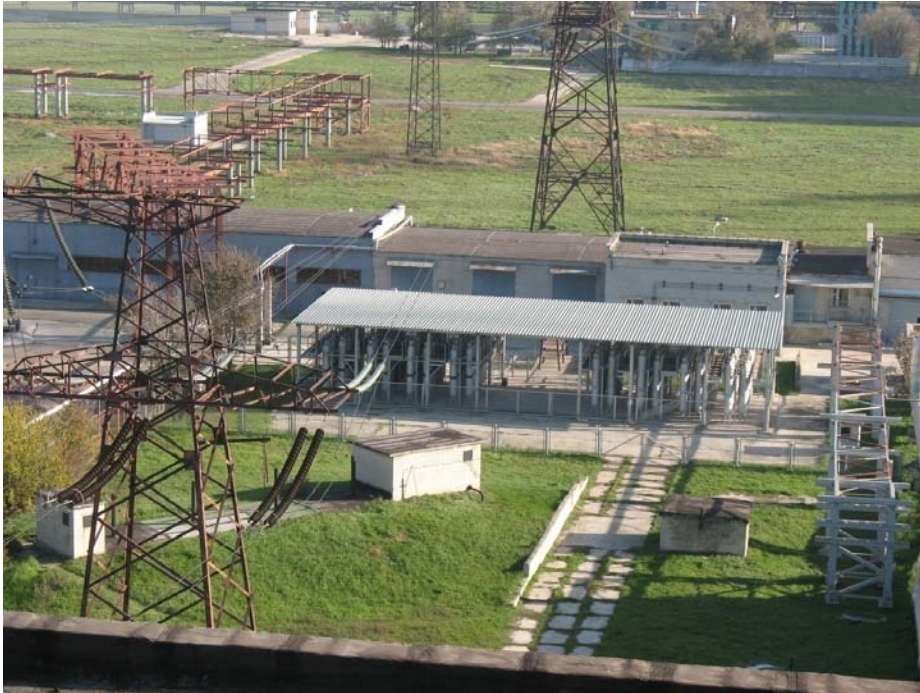
Figure 4. The nitrogen and oxygen station (open recipient arranging)
