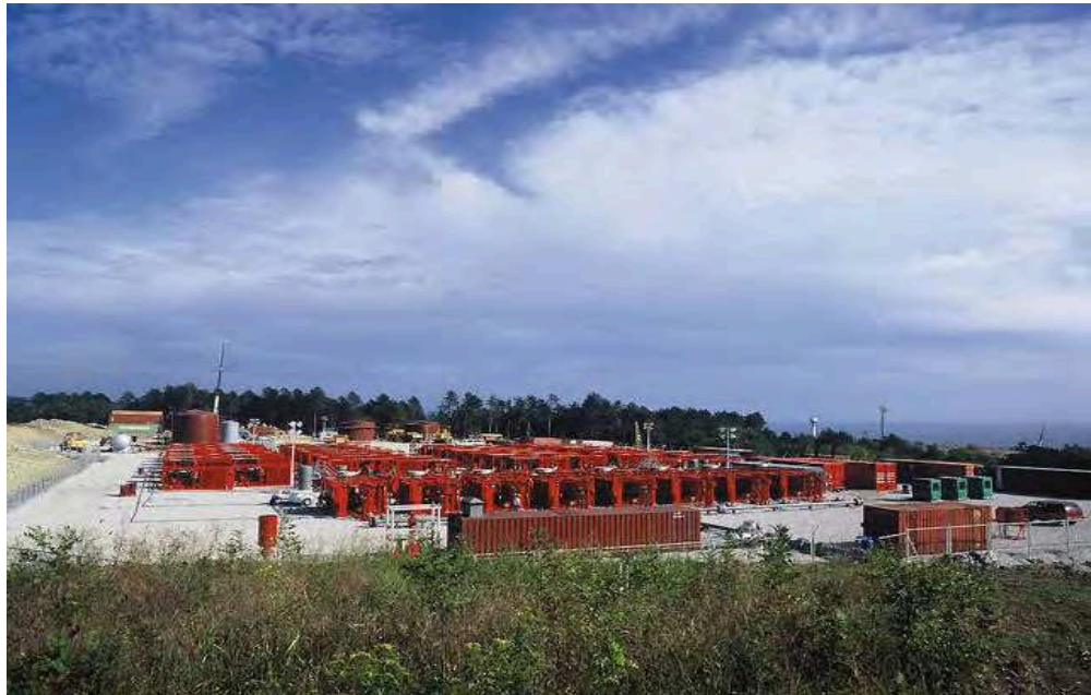
Photo 3.3 Illustration of a Typical De-watering Compressor Spread
