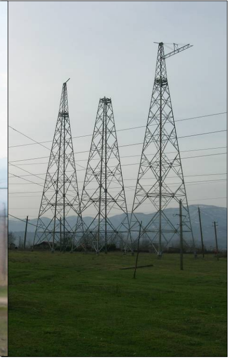
Triple 4-point contact steel lattice towers. Used primarily for direction changes and high conductor stress situations.
