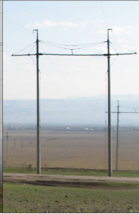
H-Frame 2-point contact tower. Used primarily for in-line conductors.
