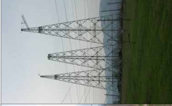
Triple 4-point contact steel lattice towers. Used primarily for direction changes and high conductor stress situations.
