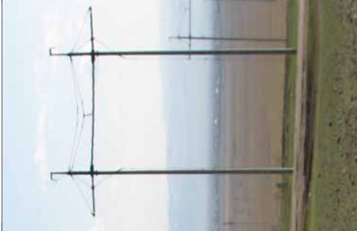
H-Frame 2-point contact tower. Used primarily for in-line conductors.
