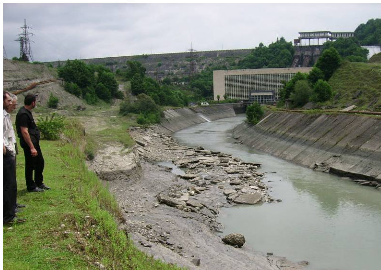
Figure A.1.1 View on landslide on right bank
