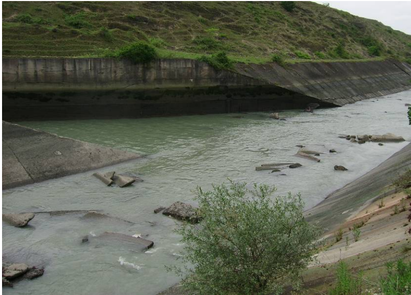
Figure A.1.3 Displaced reinforced concrete slabs
