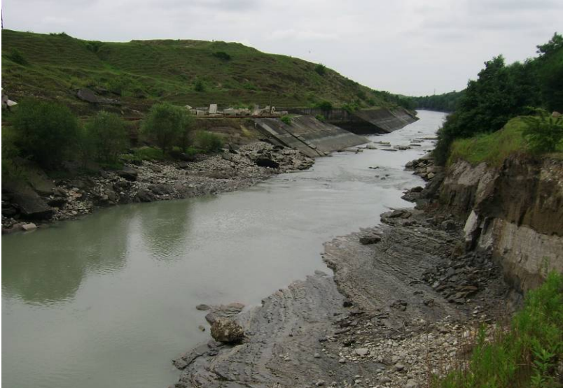
Figure A.1.2 The slopes damaged by the landslide
