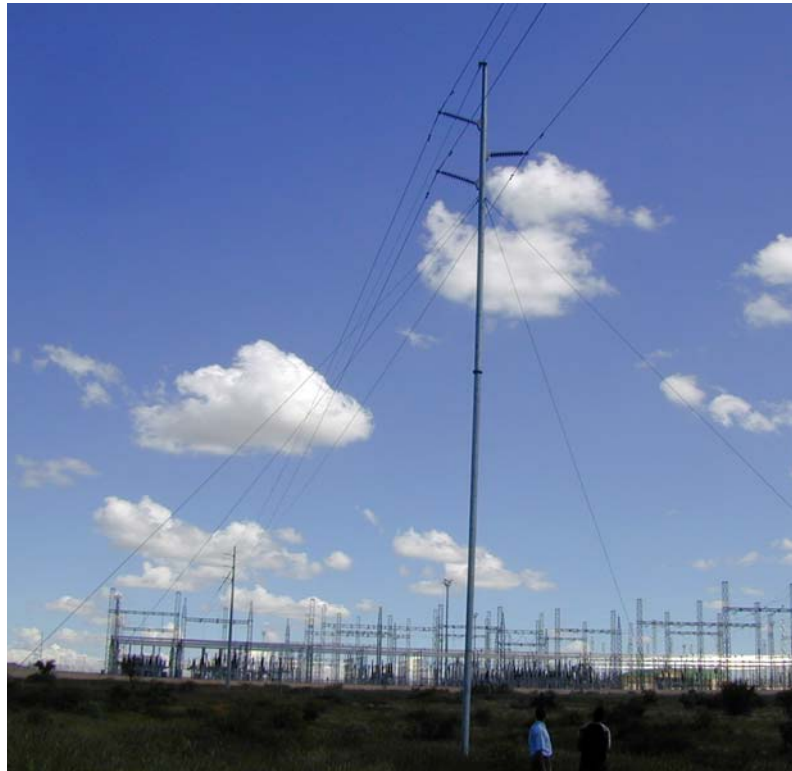
Photo 7: A typical steel tower used for a 132kV power line. These structures are not visually very intrusive, and there will be no substation such as that shown in the background to this photo.
