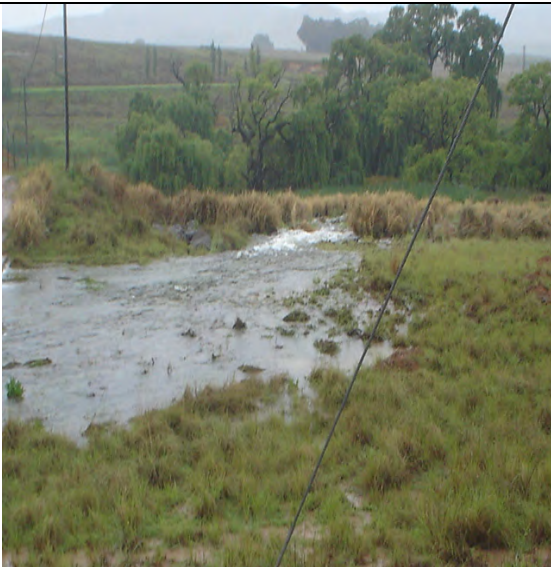
Photo 7: Overflow of the private dam moving towards the rehabilitation and erosion prevention flora ( Vertiveria zizanoides ).
