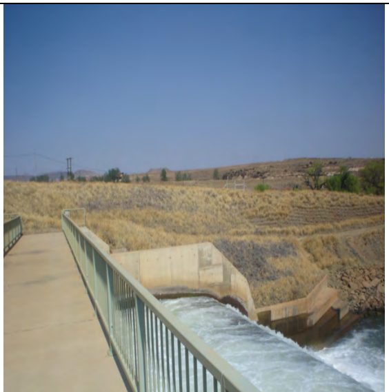
Photo 12: Narrow, 5 tonne bridge, indicating limited width.
