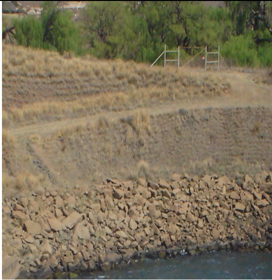
Photo 13: Disturbed dam walls which were reinforced with heavy rockfill to prevent walls from collapsing.
