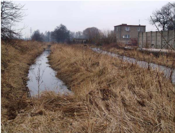
Drawing 19. PKP (Polish Railways) area draining ditch, view in the mouth direction
