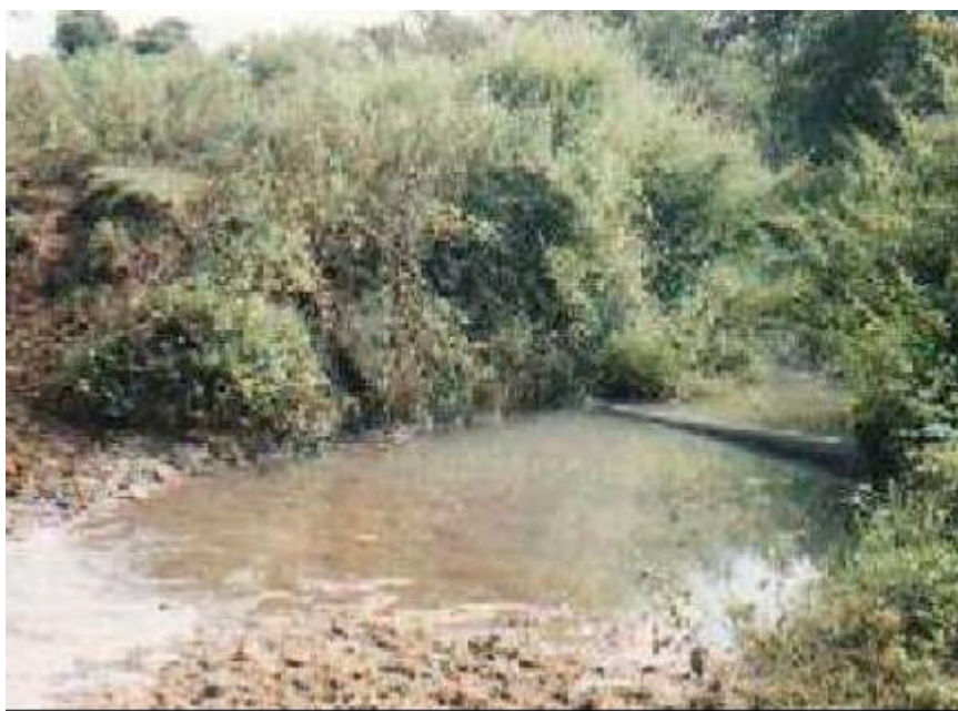
Plate 4.6: An Exposed Existing Pipeline at a River Crossing
