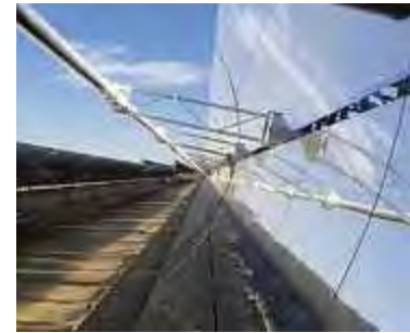
Collectors of solar thermal plant, Granada
