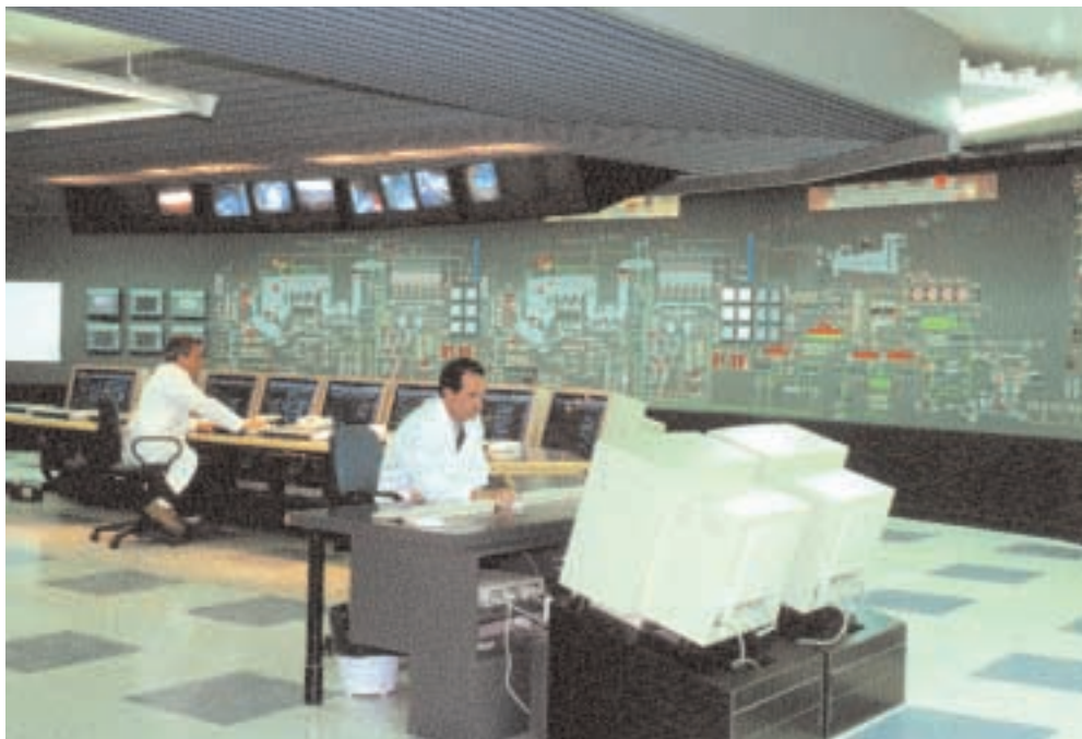
Urban waste incineration plant in Brescia, Italy
