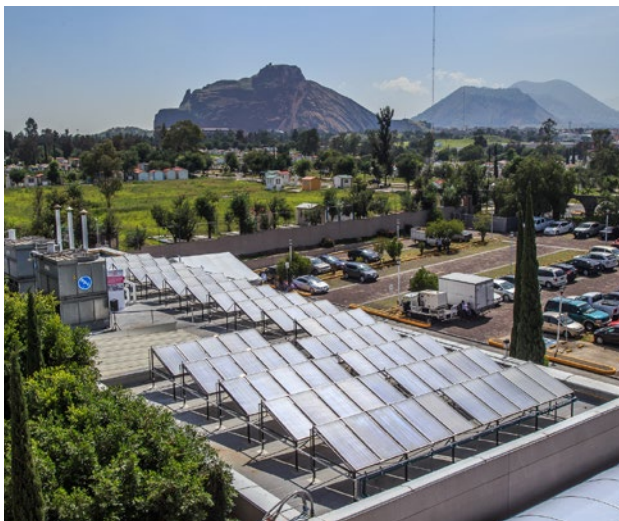
Solar Water Heaters installed on the rooftop of Public Building of Mexico City
