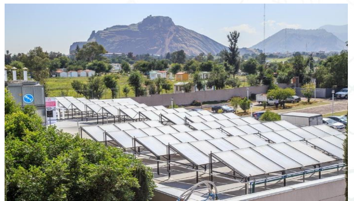
Solar water heaters installed on the rooftop of a public building in Mexico City.
