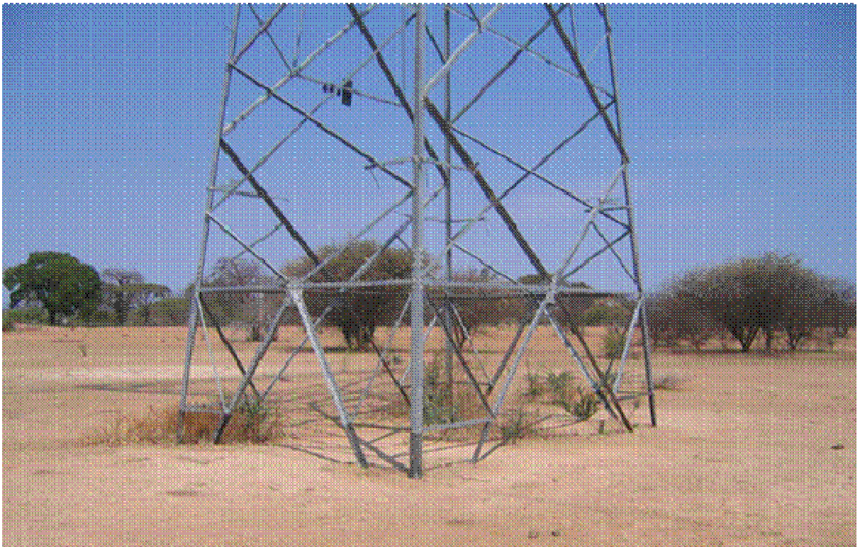
Figure 6-2: Sedimentation (near Mlowa Barabarani) Tower footing about 1m below the surface
