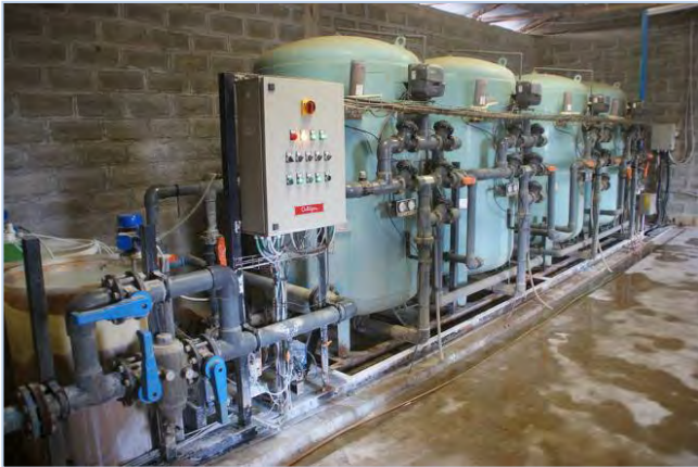
Each camp is equipped with a water supply treatment plant including flocculation (Aluminium sulfate) , filtration and chlorination
