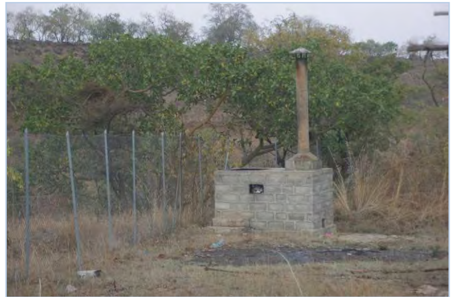
Each clinic is equipped with an incinerator for contaminated medical waste
