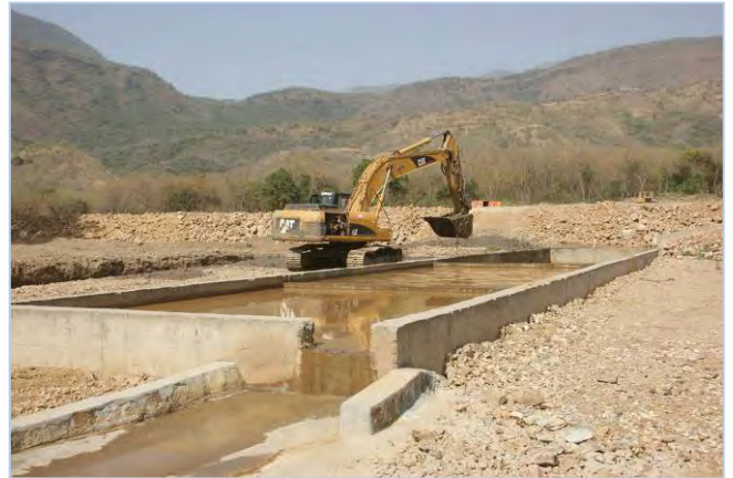
Sedimentation ponds for waste water from gravel cleaning operation. Sludge is being removed from the pond. The effluent water is discharged into a channel....
