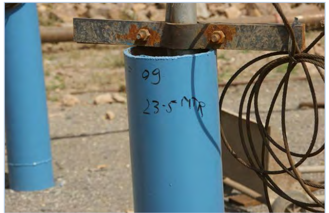
Water is pumped from a 20 to 25 m depth in the rivers alluvial aquifer
