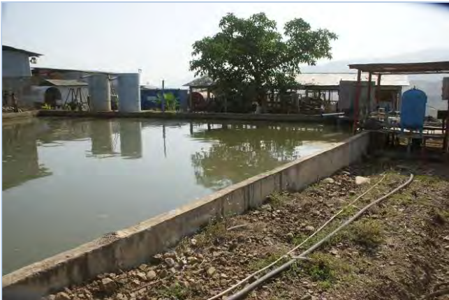
Water is pumped up into a raw water storage tank next to the Contractor's Offices from where it is pumped to the various camps
