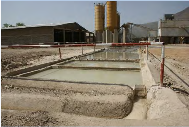
Sedimentation ponds for batching plants waste water
