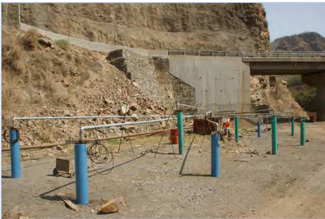
Pumping field for water supply of the camps & facilities located along the Omo River next to the new bridge (in the background)
