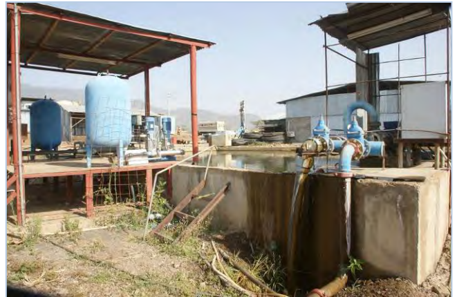
Next to the storage, a treatment plant supplies potable water to the Offices area
