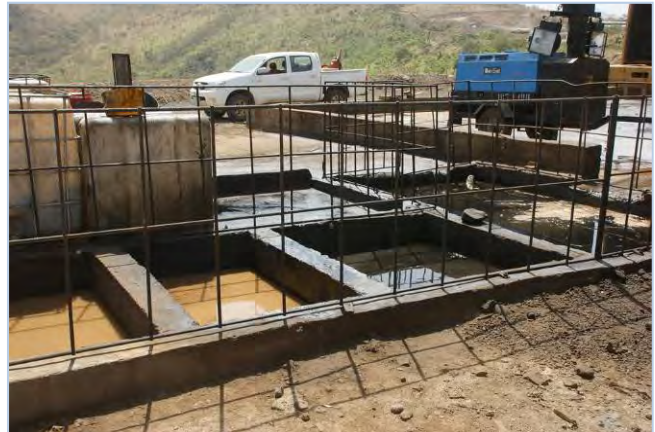
All maintenance areas are equipped with similar waste water treatment systems.
